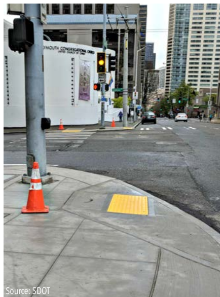
Safety outcomes can be delivered through all well-considered transportation improvements. Here, new curb ramps are provided to align as closely as possible with the sidewalks and crosswalks served.
