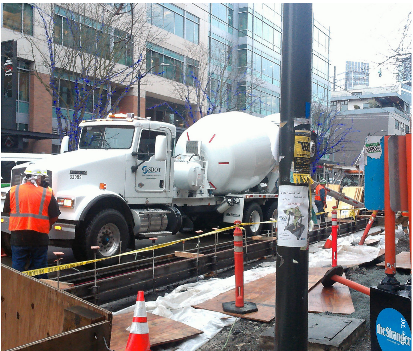
Many public and private construction projects contribute to a constrained downtown transportation system between 2017 and 2023.
